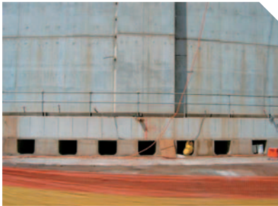
Detailed view of the bottom slab with the special accesses for BBR anchors
