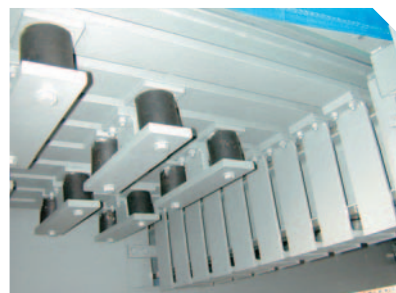
Underside of one of the expansion joints for the smaller cable-stayed bridge
